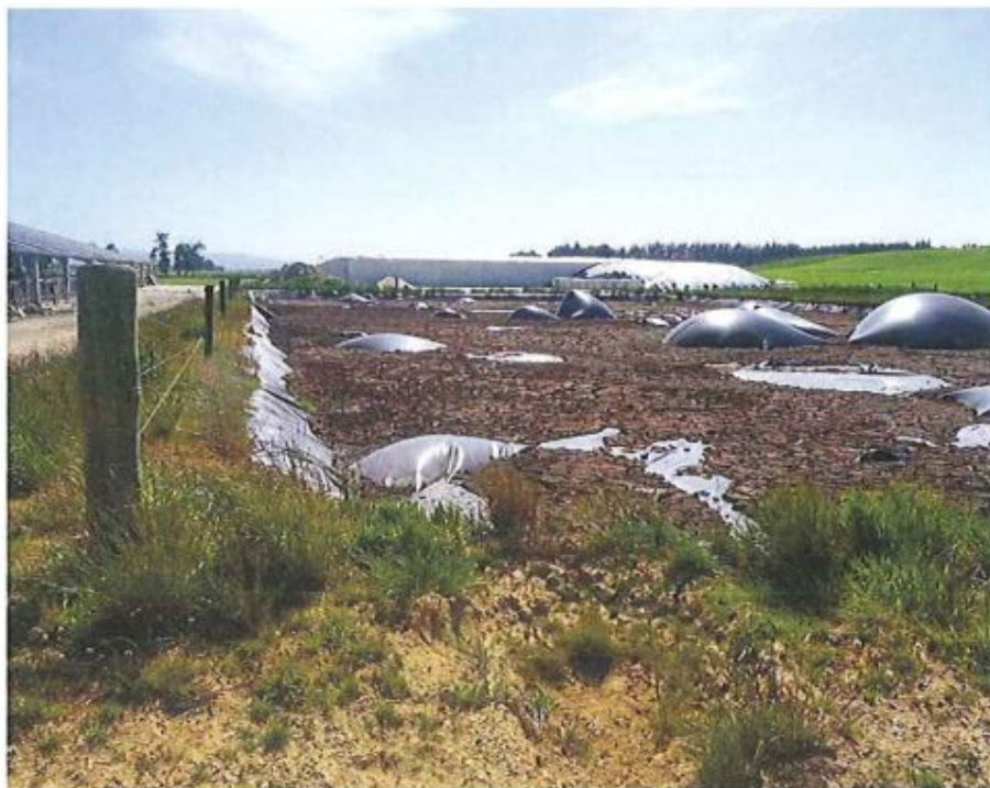
Figure 1: Incorrect gas drainage under a pond can have drastic consequences.
