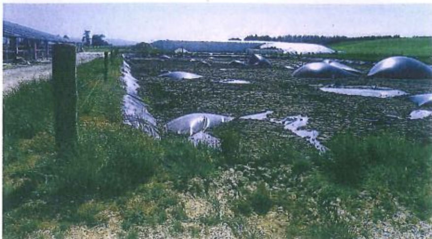
Gas hippos can develop if a drainage system has not been installed.
