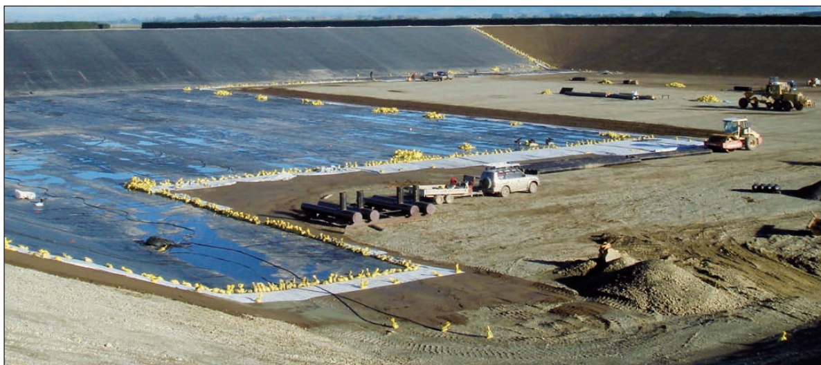
The top subgrade layer was 50mm of compacted topsoil. The Firestone 1.14mm EPDM Geomembrane liners are available in lengths up to 61m and widths to 15.25m.
